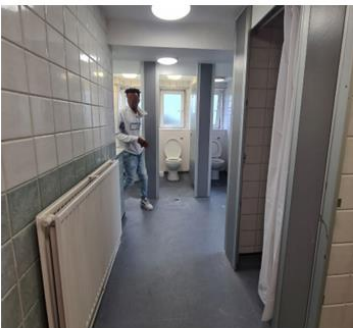
Shared WC's / bathrooms with only curtain rails providing privacy screening to shower cubicles
