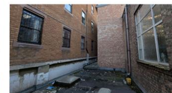
Windows to resident bedspaces with poor access to natural light and outdoor visual aspect
